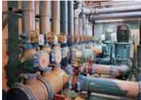
給水管 Water supply pipes
