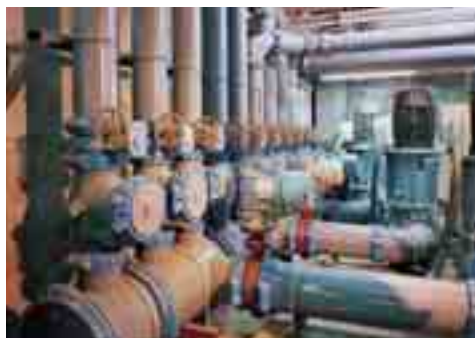
給水管 Water supply pipes
